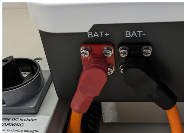
Fig 1: Underside of BPE PowerDepot Hybrid Inverter, with battery leads connected.
